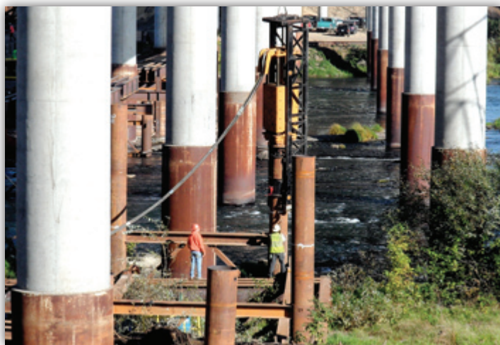
Hydraulic mechanisms at WRB use canola oil instead of petroleum-based products to reduce risk to the environment. The amount of oil it takes to cook your Holiday turkey will keep this impact hammer going for about six months. (from left) Veril Humbert and Mike Sheeley running the Hydraulic Impact Hammer while building work bridge.
